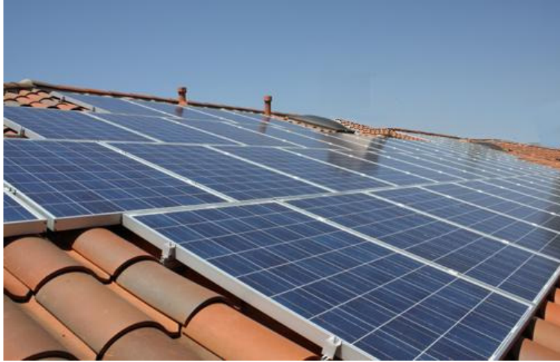
12.5KW Grid Solar Power System in Southern California (Residential)
