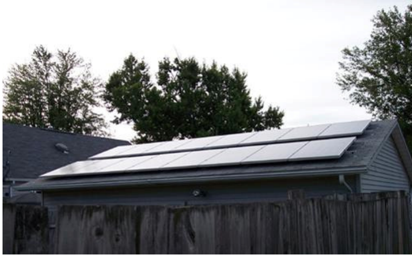
3.2KW Grid Solar Power System in Mid west (Residential)
